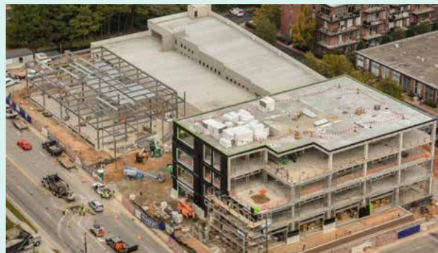
Figure 15: Chamblee Station is where a local developer is building a 70,000 square foot office building with 10,000 square feet of retail on a two-acre parcel owned by MARTA. The parcel is directly adjacent to Chamblee Station.
